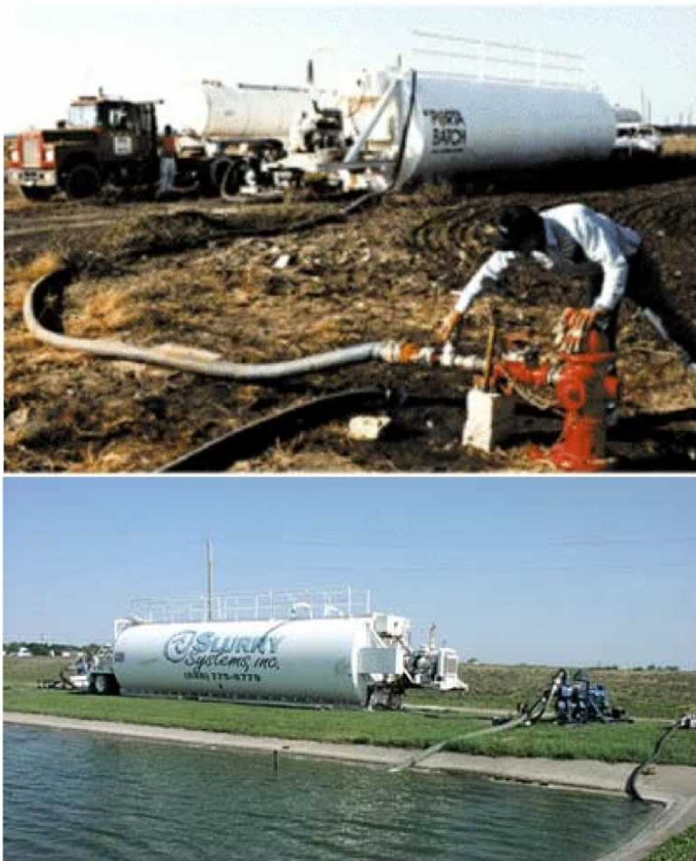
Figure 6: Portable lime slaker tanks for preparing lime slurry on-site
