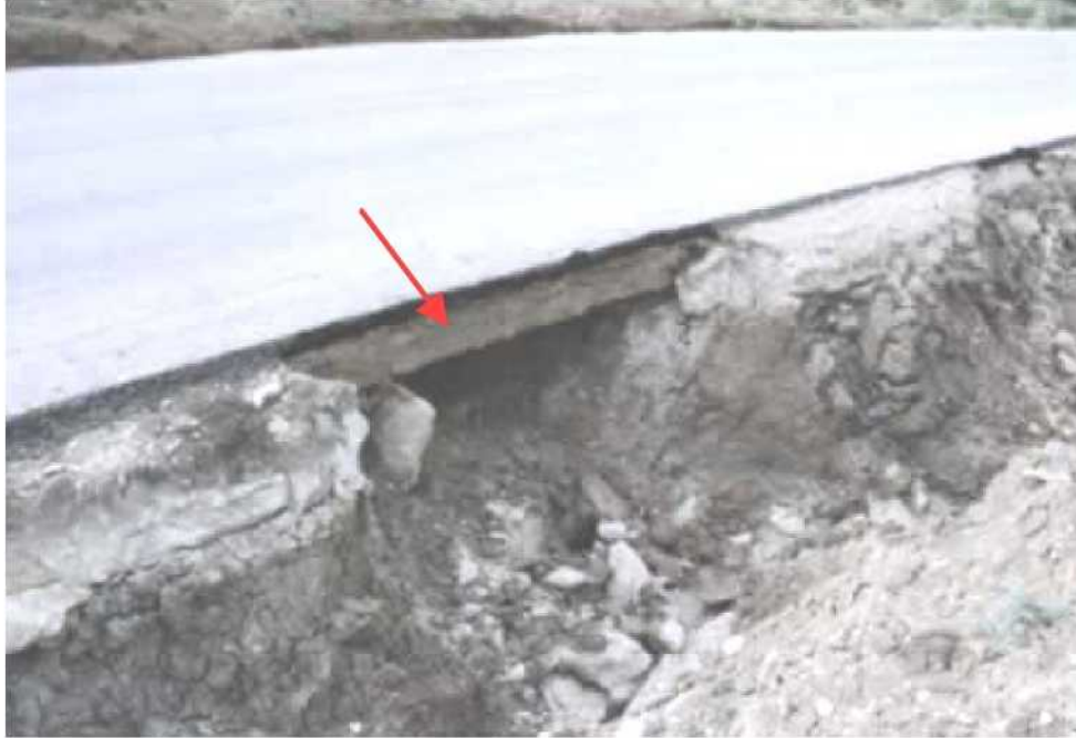
Figure 3: Lime-stabilized layer (see arrow) bridging an erosion failure illustrates strength
